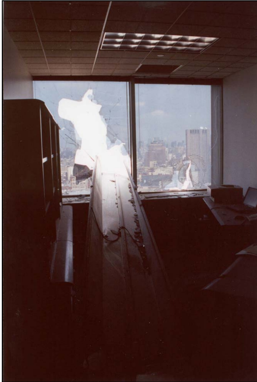
Figure 7a. Office space damage above tenant level 29 — penetration of tower 2 fascia piece.
