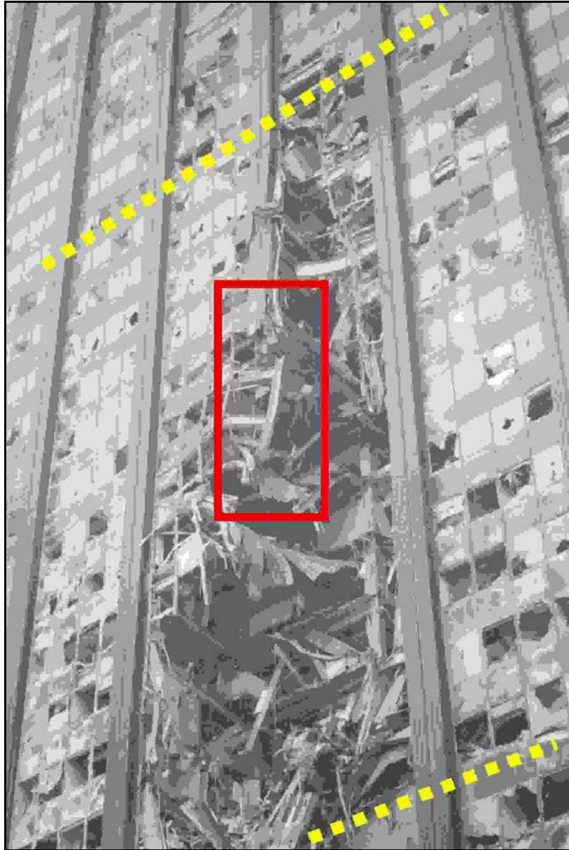
Figure 12a. Damage to the northern face of the building between tenant levels 23 and 10—view of damage zone between levels 23 and 10.
