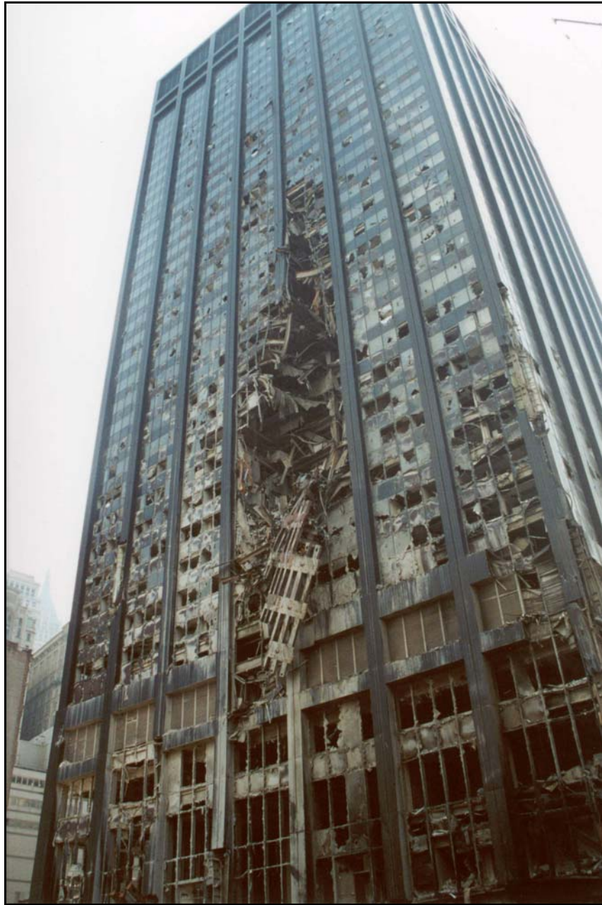
Figure 4a. Damage to the 130 Liberty Plaza building from the exterior—view of northern façade.
