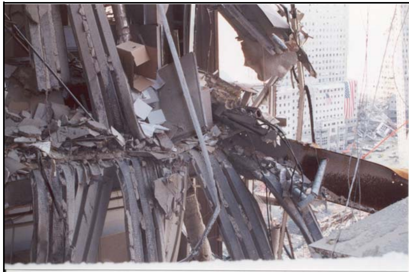
Figure 10b. Interior damage photographs from tenant level 19— floor framing on line 8 between lines C and D.
