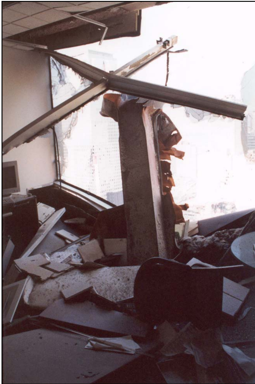
Figure 8b. Damage due to column-missile ejected from tower 2—upper end of column-missile above level 29.
