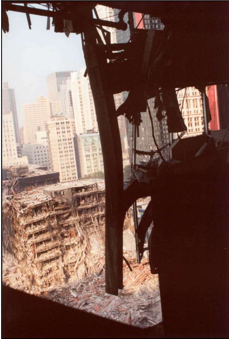
Figure 11b. Fractured column on line D from tenant levels 18 and 17—view at level 17.
