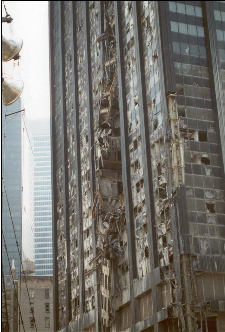
Figure 4b. Damage to the 130 Liberty Plaza building from the exterior—view of northern and western facades.
