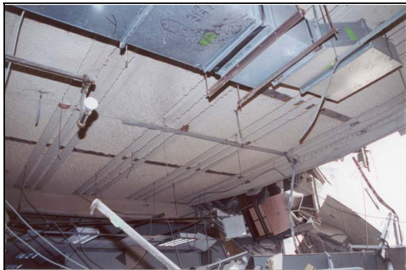
Figure 9b. Interior damage at tenant levels 22 and 21—underside of level 22 slab looking northwest.
