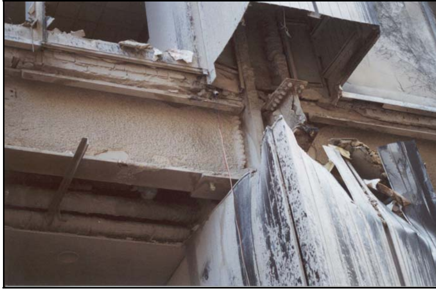
Figure 5b. Exposed steel moment framing in the first story of the building—first story of the western face.
