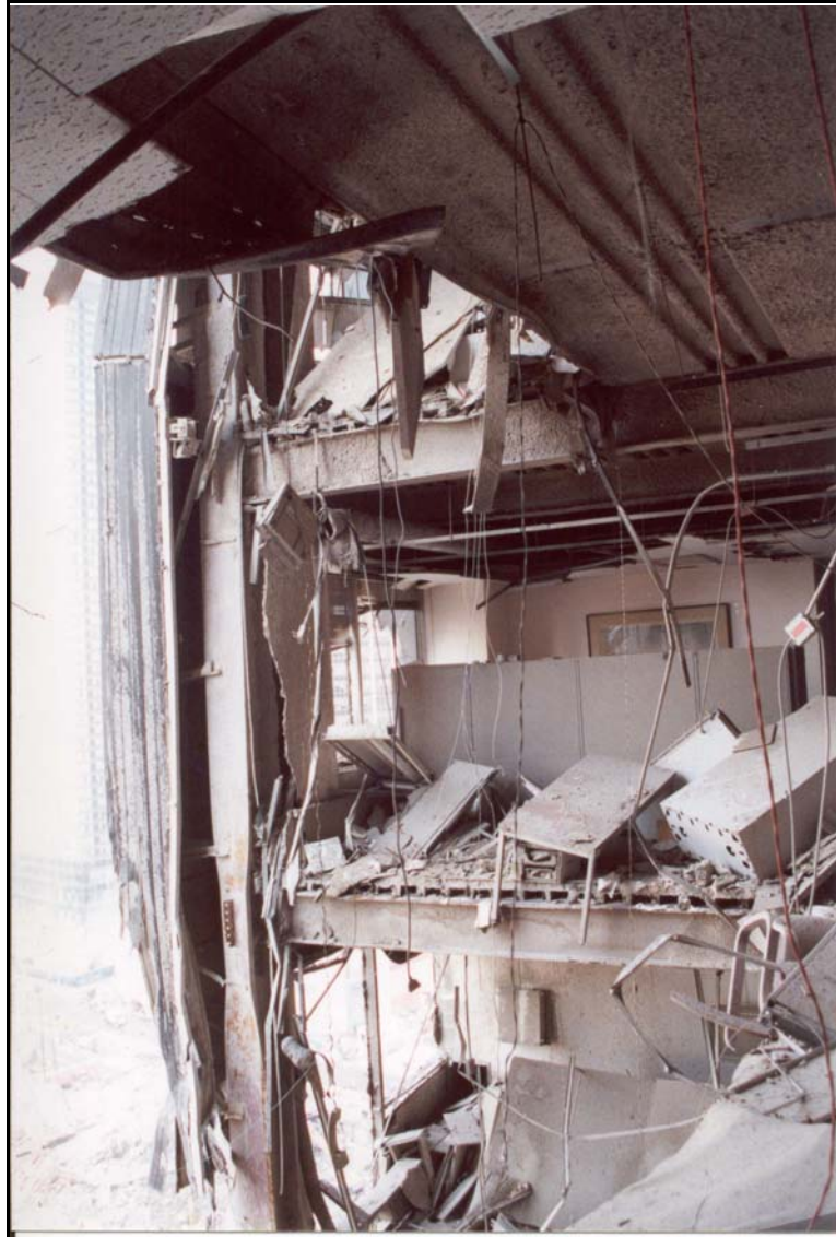
Figure 10c. Interior damage photographs from tenant level 19— damaged framing at levels 19 and 20.
