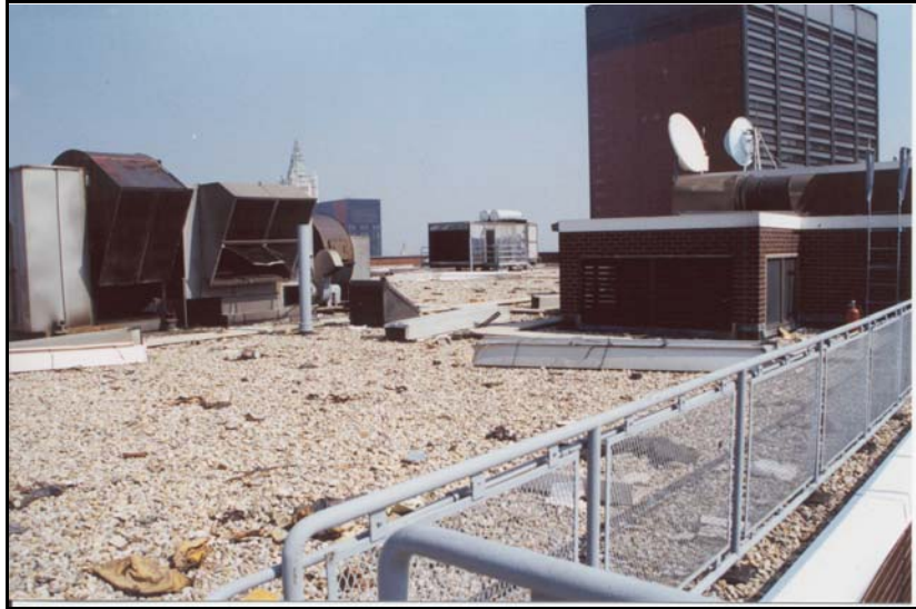
Figure 6a. Debris at the roof level of 130 Liberty Plaza— photograph looking east.
