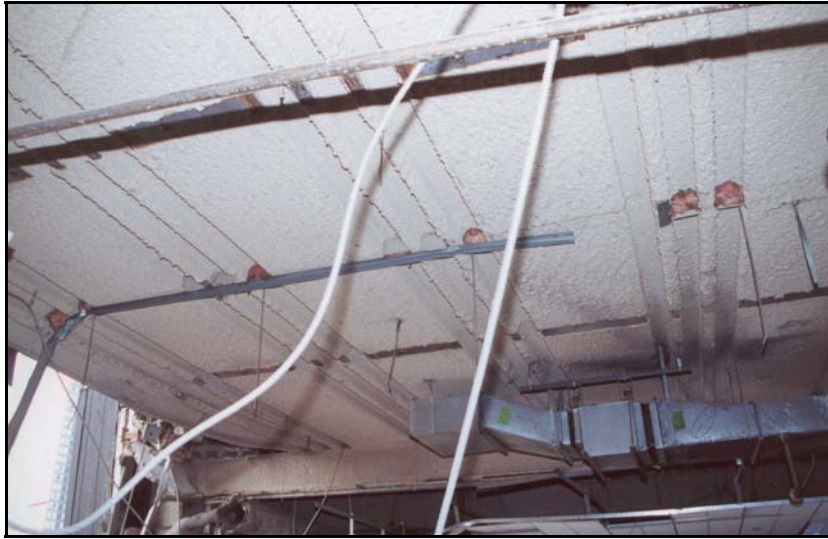
Figure 9c. Interior damage at tenant levels 22 and 21—underside of level 22 slab looking northeast.
