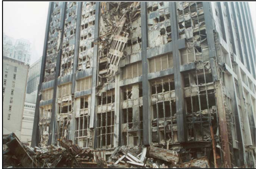
Figure 4c. Damage to the 130 Liberty Plaza building from the exterior—view of lower 10 stories of northern façade.
