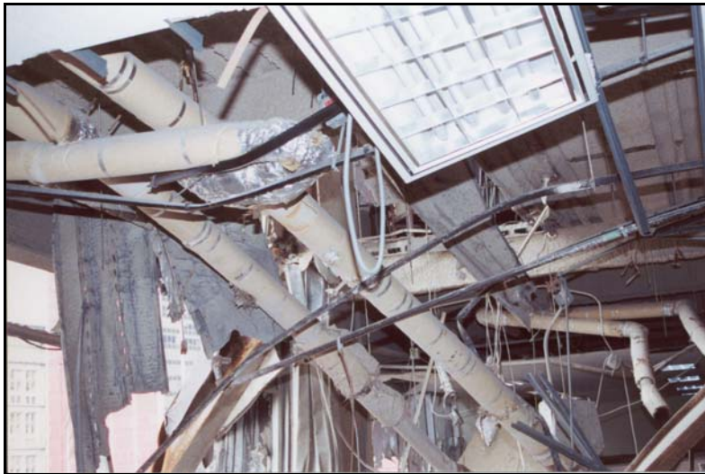
Figure 9d. Interior damage at tenant levels 22 and 21—underside of level 21 slab looking northeast.
