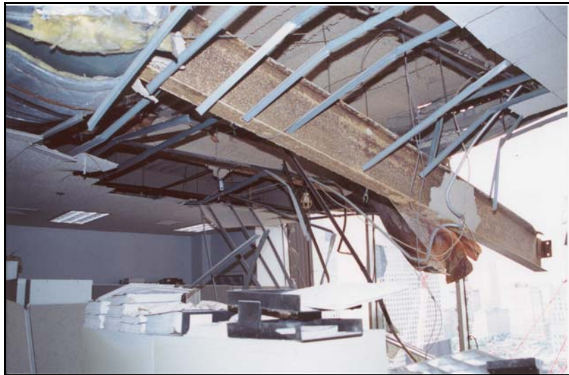
Figure 9a. Interior damage at tenant levels 22 and 21—underside of level 23 slab looking northwest.
