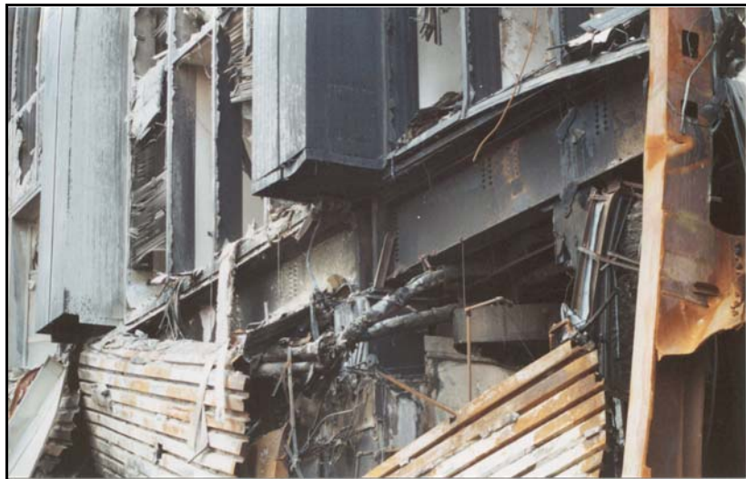
Figure 5a. Exposed steel moment framing in the first story of the building—first story of northern face.
