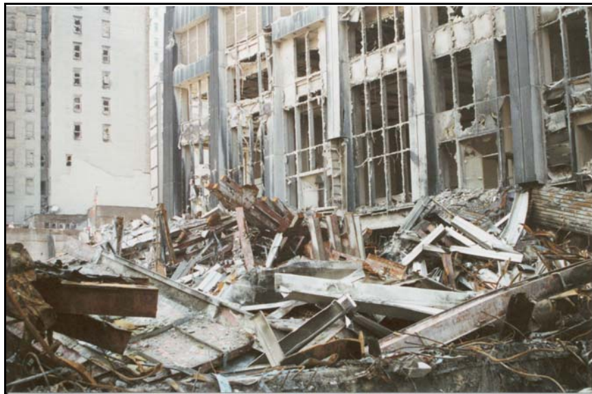
Figure 4d. Damage to the 130 Liberty Plaza building from the exterior—damage to northern façade at the entry level.
