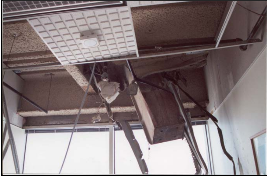
Figure 8c. Damage due to column-missile ejected from tower 2— Lower end of column-missile below level 29.
