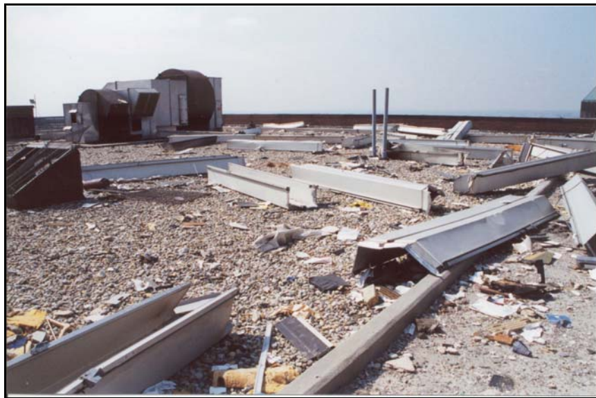
Figure 6b. Debris at the roof level of 130 Liberty Plaza— photograph looking west.
