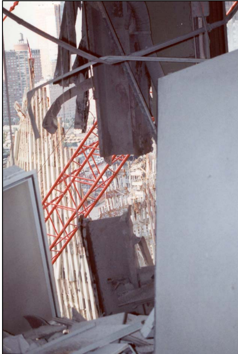
Figure 11a. Fractured column on line D from tenant levels 18 and 17—view at level 18.
