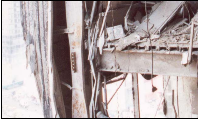
Figure 10a. Interior damage photographs from tenant level 19— failed moment connection at grid D8.
