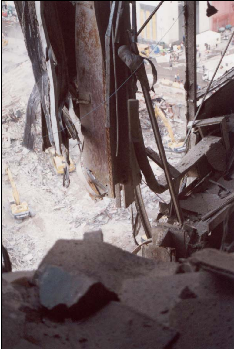
Figure 10d. Interior damage photographs from tenant level 19— failed column immediately above level 18.
