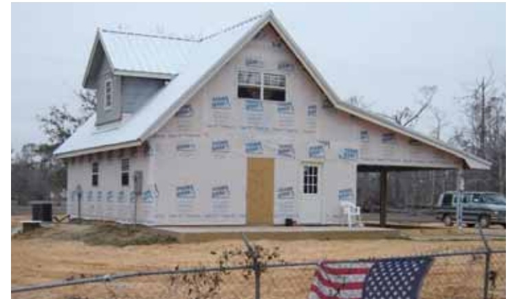
Oct. 2006 Waveland, MS Source: Hazards Research Lab
