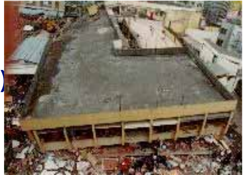
A building collapsed in Taipei Basin with ED >100 km (Hwa-lian EQ, 1986)
