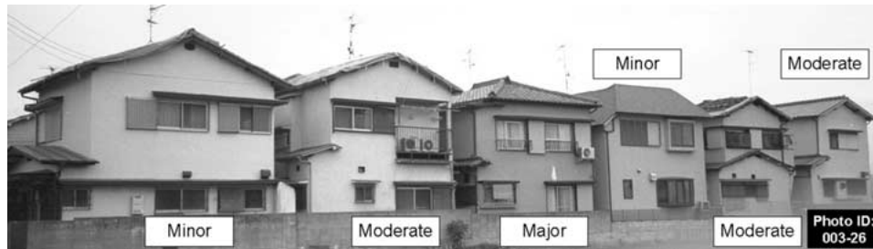
Photograph 1. Actual example of results in Housing damage assessment .
