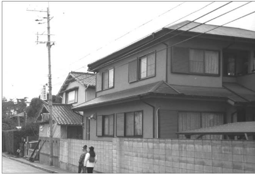
Photograph 3. Example of limitation of visual inspection from outside (result of assessment for Victim Certificate: Major damage).
