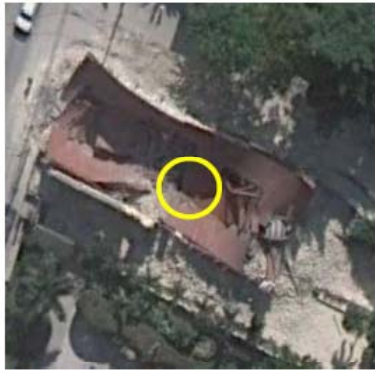
Level 5 - Destruction: All or most of building structure collapsed. Here: Collapsed/broken roof, walls destroyed (debris surrounding building)
