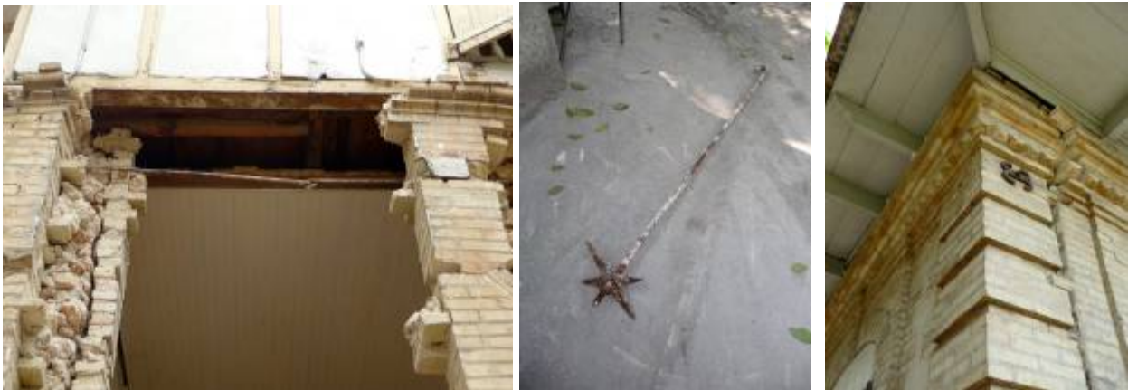
Fig. 11. Iron tension rods. Left – Linked rods exposed. Limestone infill panel was discharged. Tension rod may have prevented complete wall collapse. Center - End rod isolated, showing hooked end and threaded end with star plate and nut. Right - Brick corner with one end plate missing, showing separation of corner pier from rest of wall in that direction.
