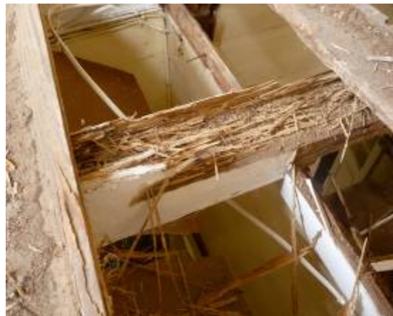
Fig. 32. Termite damage in second story floor joists.
