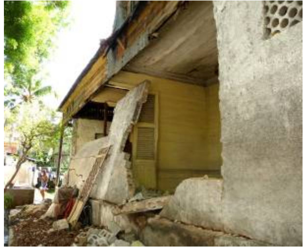
Fig. 25. A replacement side wall of concrete block suffered partial collapse. (19 Lamartiniere)
