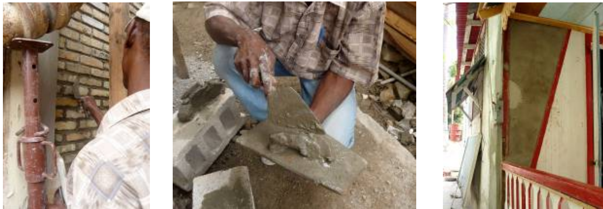
Fig. 32. Well-intentioned but improper repairs with cement mortar in brick work (left and center), and cement plaster for colombage infill (right). Lime mortar and lime plaster should be used.
