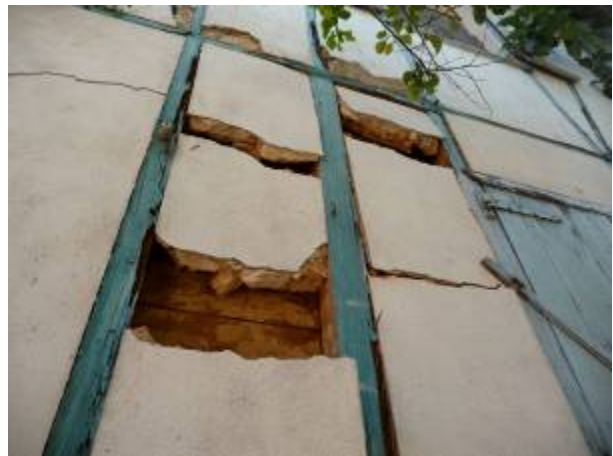
Fig. 13. Colombage with limestone and earth mortar infill, with lime plaster finish. Interior planking can be seen. (5 Rue Jose Marti)
