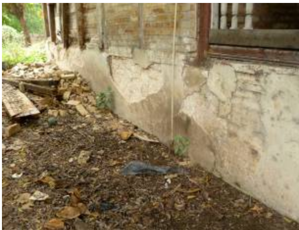
Fig. 17. Spalling of the exterior finish plaster reveals two contiguous sections of foundation stem wall. One of irregular limestone (left), and one of brick (right). (84 Lamartiniere)
