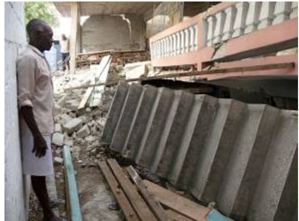
Fig. 27. An expansive two-story, concrete classroom addition behind the original building suffered first story collapse.
