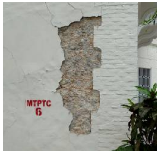
Fig. 10. Delamination of finish plaster reveals the limestone infill panel bounded by the corner brick pier. MTPTC 6 indicates inspection deemed tower unsafe for occupancy.
