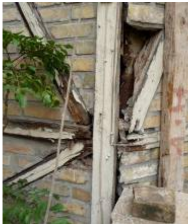
Fig. 31. Rot of timber frame members at corner of colombage house. (32 Lamartiniere)
