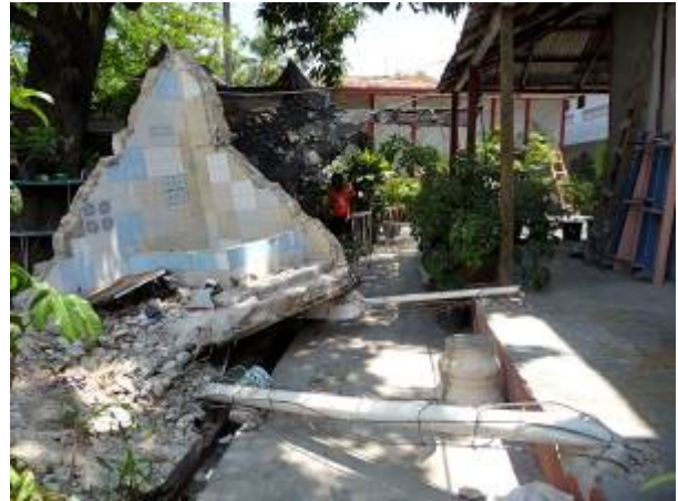
Fig. 28. This second floor concrete bathroom addition landed on the ground after its concrete columns buckled as it pulled away from its parent gingerbread house. Note sewer pipes in the center of the rebar of the buckled columns. (5 Lamartiniere)
