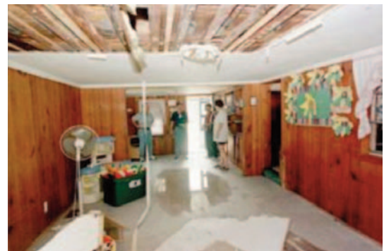
Source: Federal Emergency Management Agency, photograph taken by Dave Gatley of FEMA. Moisture damage is not just related to flooding. Here, an inspector is seen evaluating water damage when a roof was compromised by wind and rain.
