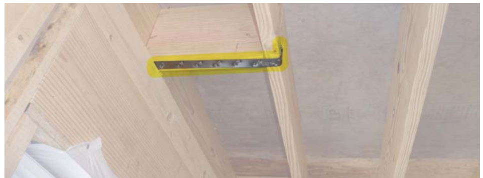
$20 worth of standard twist straps and coil strapping from a local hardware store were used to correct a new failure mode identified during the wind test demonstrations.
