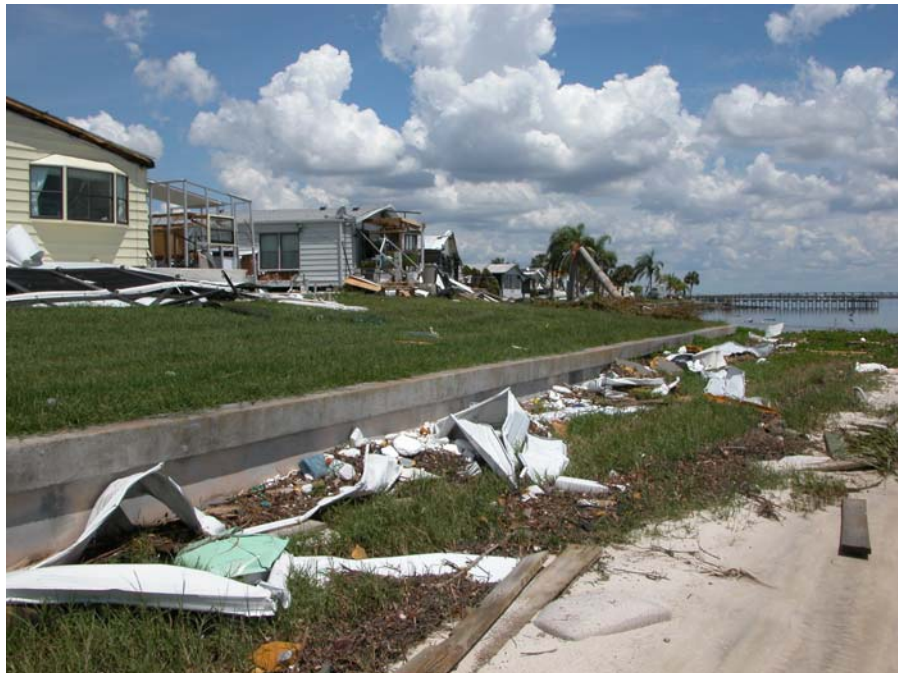
Figure 7. Harborview Park's location and damage.
