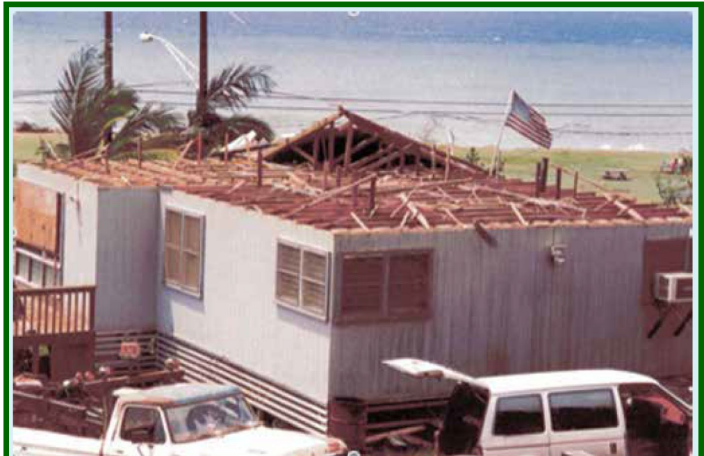
Figure 2-5. A common site on Kaua'i after Hurricane Iniki. Many roofs were blown off due to a lack of proper connection. Photo courtesy of Department of Commerce and Consumer Affairs Insurance Division.
