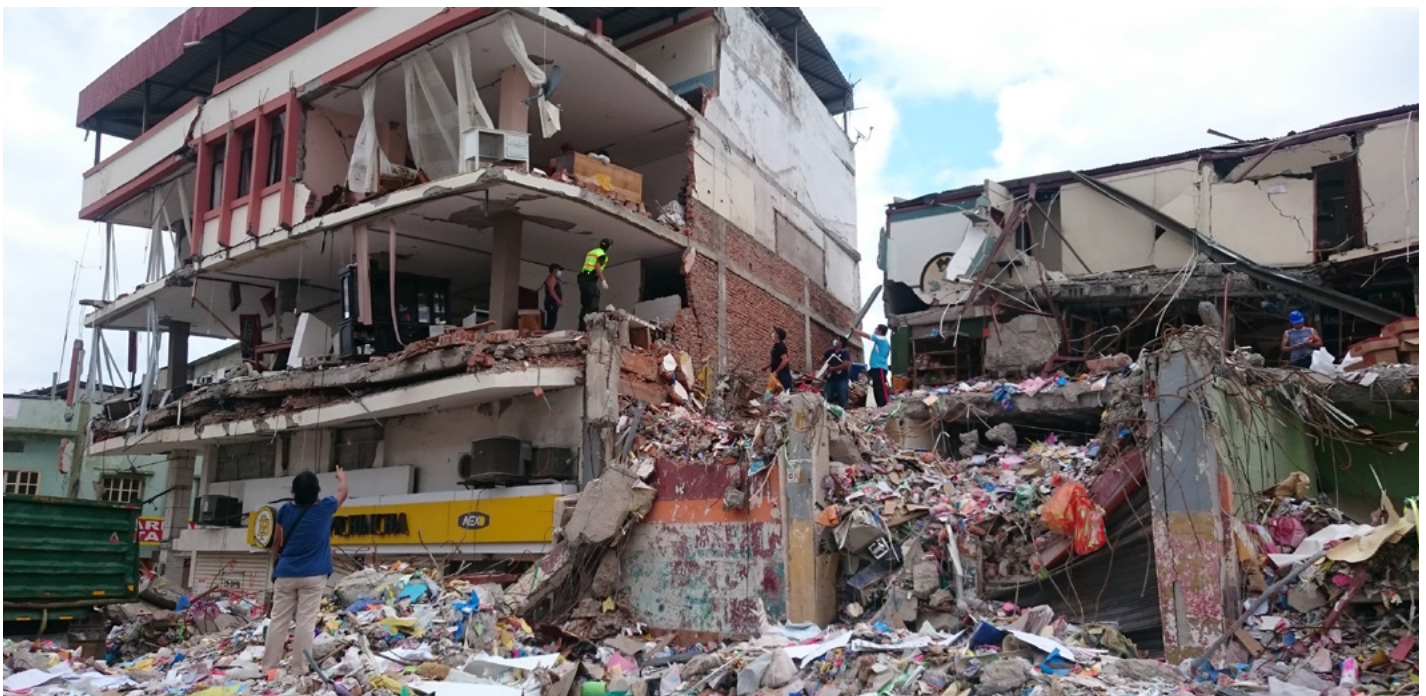
Figure 1. In Manta, Ecuador, one of the worst affected cities, the entire neighbourhood of Tarqui was destroyed. © European Union/ECHO, 2016
