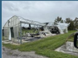
Preliminary damage assessments following Hurricane Milton in Florida
