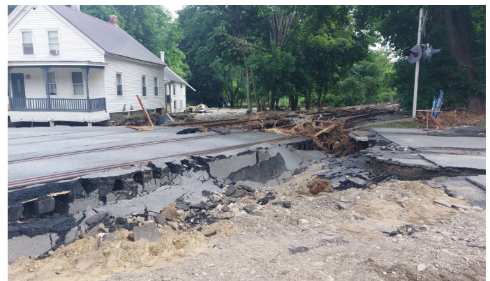
A house and railway in Proctorsville, Vermont that were damaged during acute flooding in July 2023. Photo credit: Charis Boke, 2023.
