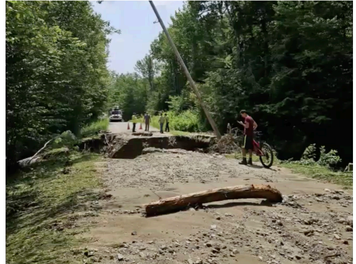
A normally small stream surged with water during the flood, eroding all roadway material around a culvert and creating a 12-foot crevasse that made the road impassable. Photo credit: Tim Banker, 2023.
