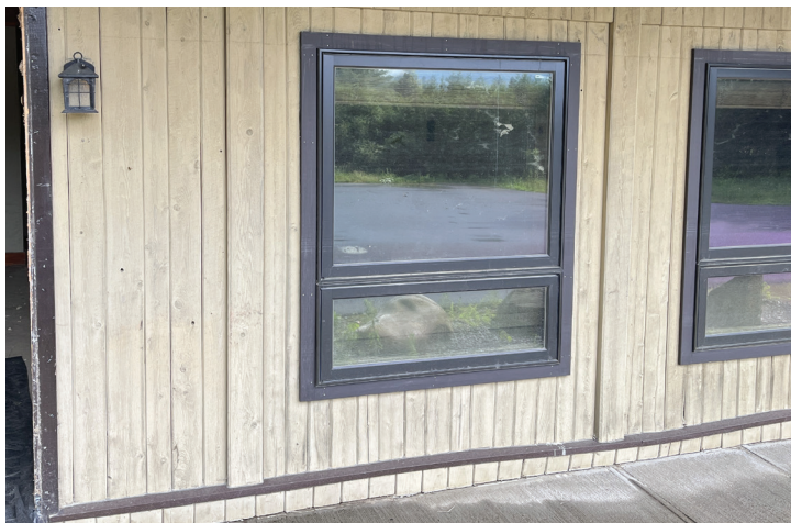
Ground floor of the Timber Inn in Ludlow, Vermont. The high-water line of the July 2023 flood can be seen at the top of the windowsill. Photo credit: Noah Bezanson, July 17, 2024.
