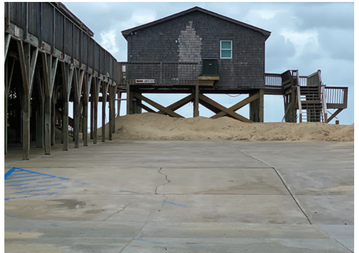
The Outer Banks Motel's individual mitigation measures included elevating HVAC and motel rooms and installing sandbag and dune barriers. ©Brianna Castro, 2020.
