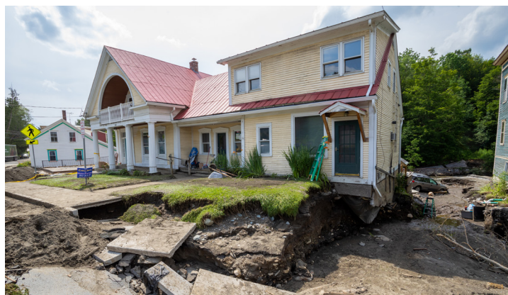
July 2023 flash flood damage to a home on the Winooski River, in nearby Cabot, Vermont. Photo credit: Mike Hardiman / Shutterstock.com
