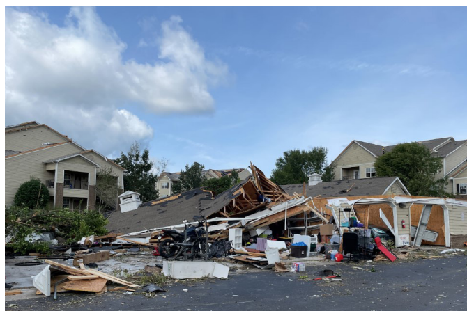
A collapsed garage after the EF-2 tornado in Knox County, Tennessee. Source: National Weather Service Tornado Storm Damage Survey, 2023.
